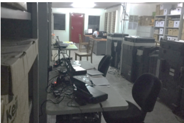
Inside view –Data-centre in the EO compound with secure server room at the end.
